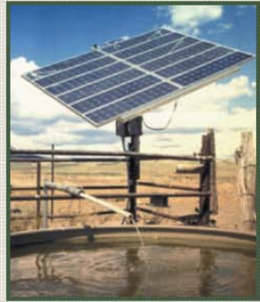
Ute Mountain Indian Reservation solar water pumping
